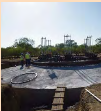
Ventika Wind Farm
